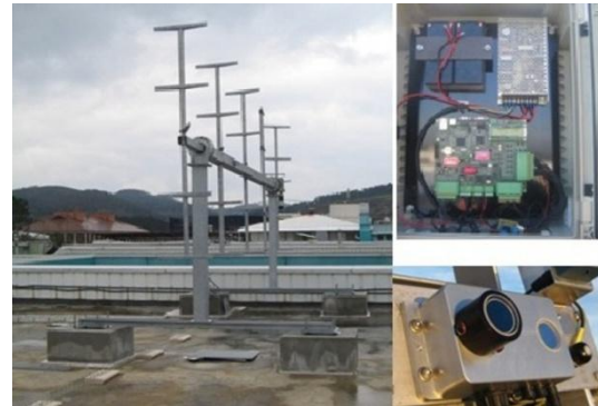
Fig.10: Tracker designed by CPower and electronic control unit developed by Tecnia, in the site of Tecnia, in Bilbao (ES).
