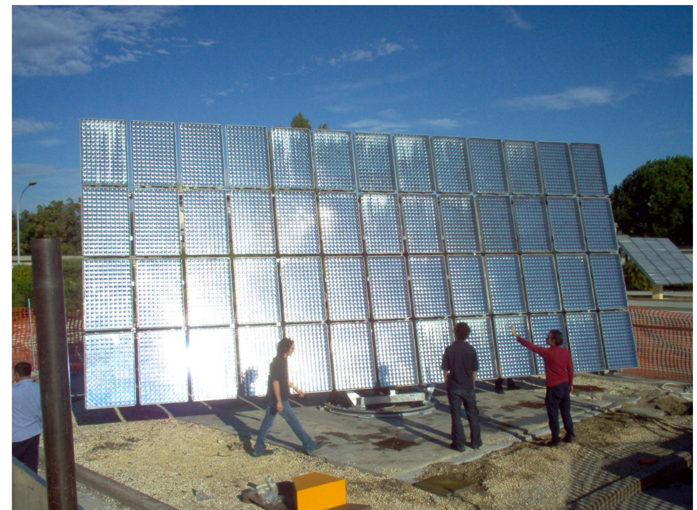
CPV prototype installed in Enel Advanced Solar Laboratory
