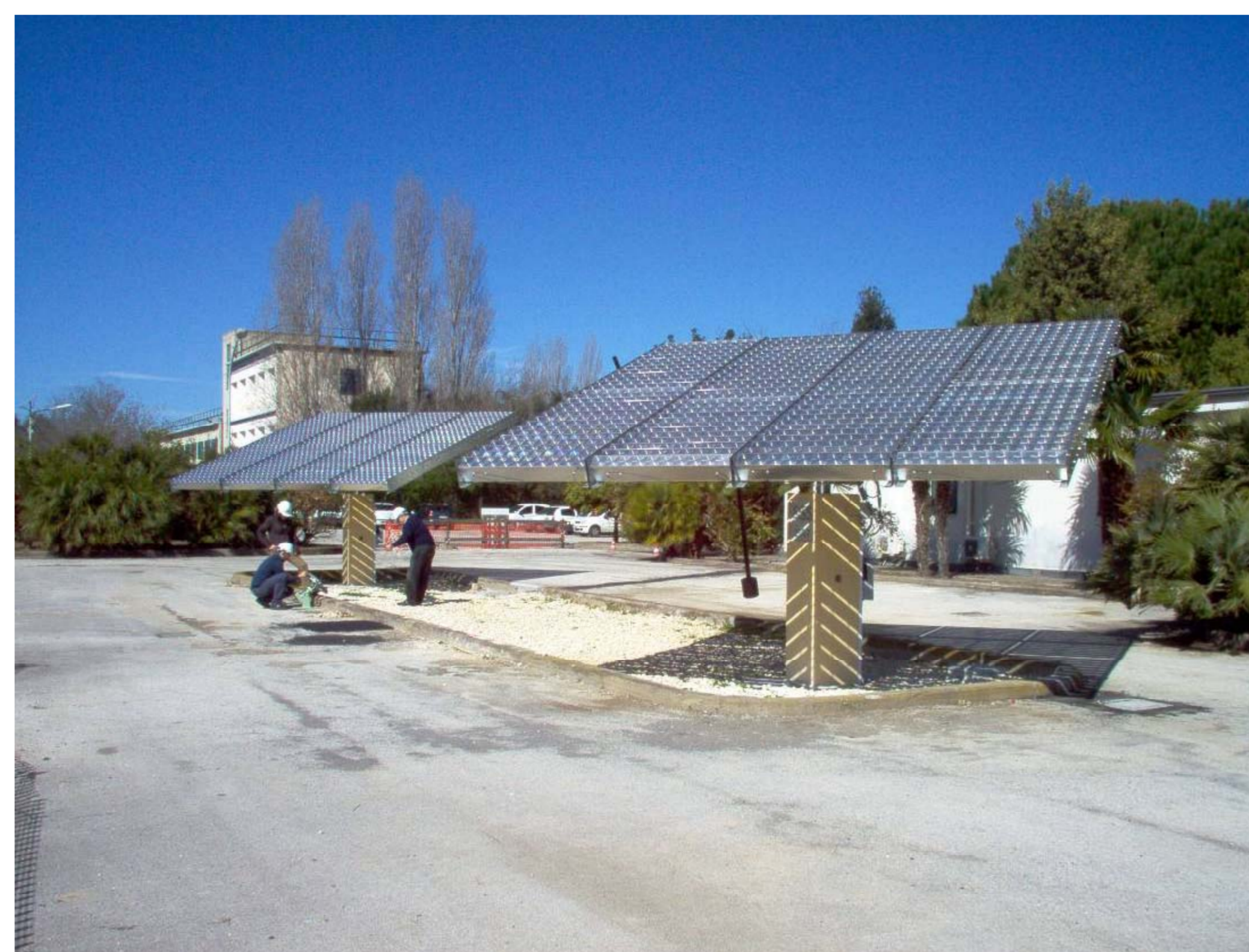
CPV prototypes installed in Enel Advanced Solar Laboratory
