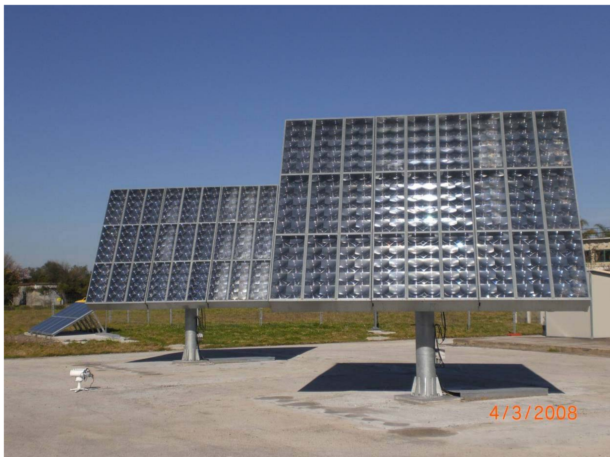
CPV prototypes installed in Enel Advanced Solar Laboratory
